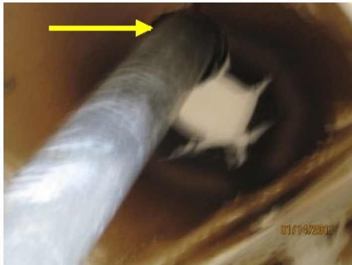
vent pipe clearance around combustable materials should be a least 1 inch
