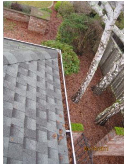
remove debris, no gutter guards
