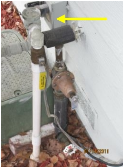
watertight cover needed for outlet
