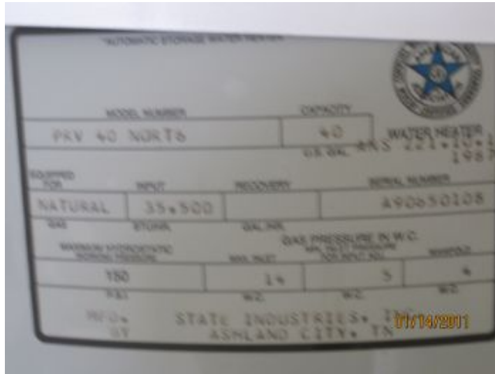
water heater reaching end of life span (1987)
